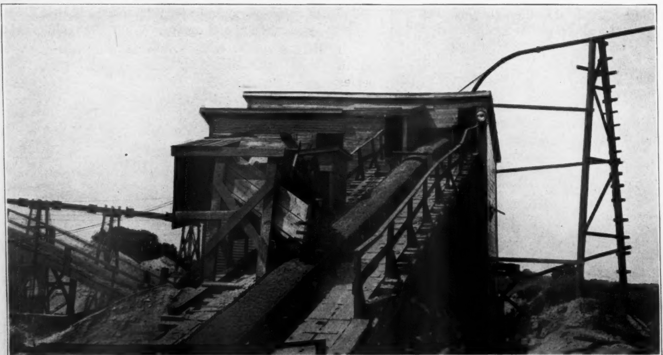
Looking Up Number 1 Belt, Crushed Material Falling on Raw Material to Scalper
